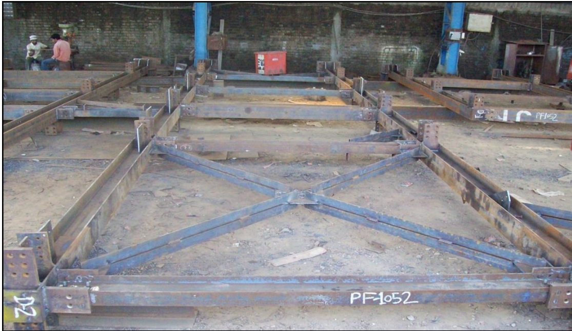
BOLTED STR CAIRN ENERGY
