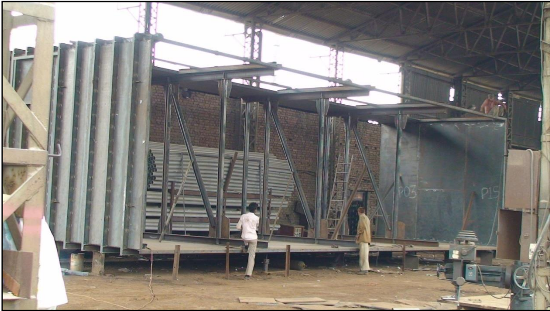
DUCT L & T
